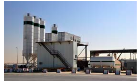
Ice store S 60 and two ice generators I 90 in Riad/Saudi-Arabia
